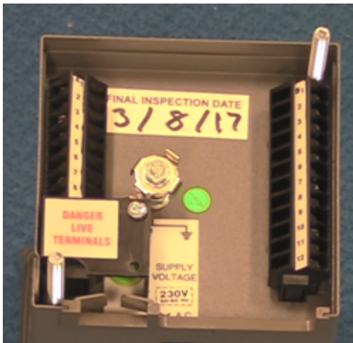
Figure 4 Power supply cover removed
